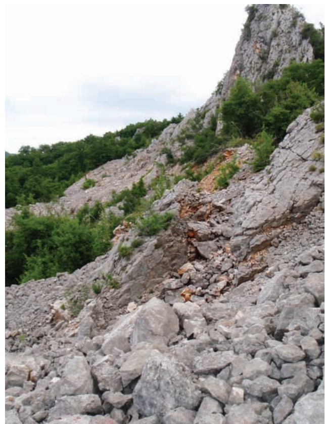
Figure 11: New open fracture on the higher eastern part of the slope (photo: BENAC, Č.).
