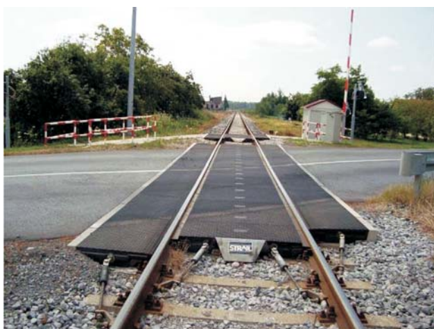
Figure 8 Renewed level crossing at km 25+700 near train stop Antunovac Slika 8. Obnovljeni cestovni prijelaz u km 25+700 ispred stajališta Antunovac
