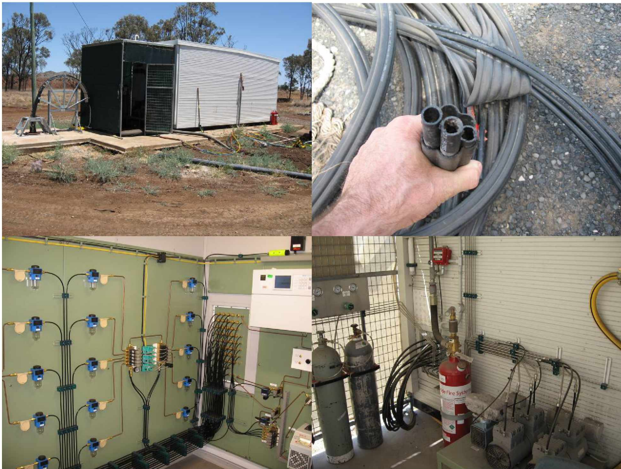
Figure 8.—Continuous atmospheric gas monitoring system in Australia. Top left: Monitoring shed over mine showing borehole and sample tubes. Top right: Close-up of sample tube bundle. Bottom right: Sample tube pumps. Bottom left: Inside monitoring shed showing manifold and gas analyzer.
