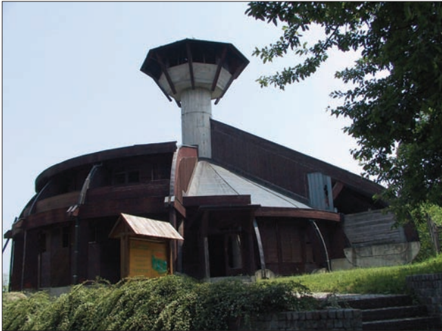
Slika 8. Devastirana zgrada. Figure 8 The devastated building.
