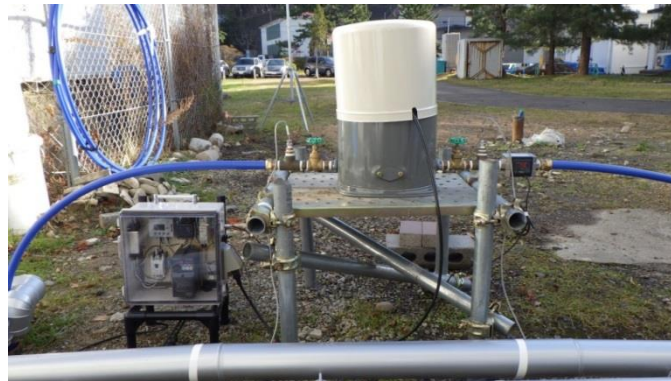
Fig. 3-6 Water pump and controlling unit.
