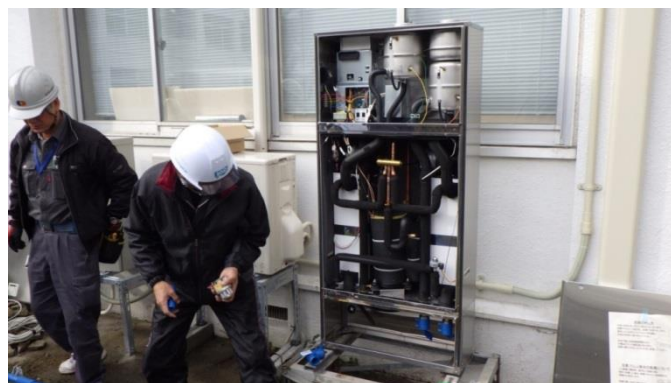
Fig. 3-7 Heat pump unit.
