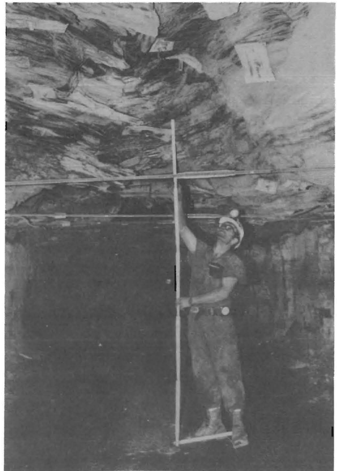
Figure A-4. —Typical intersection roof fall exhibiting stress-related shear failure.
