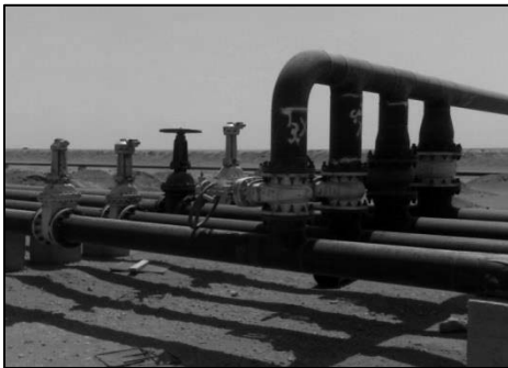
Figure 15: Pipes of the Hot Flare, Nasiriyah Degassing Station
