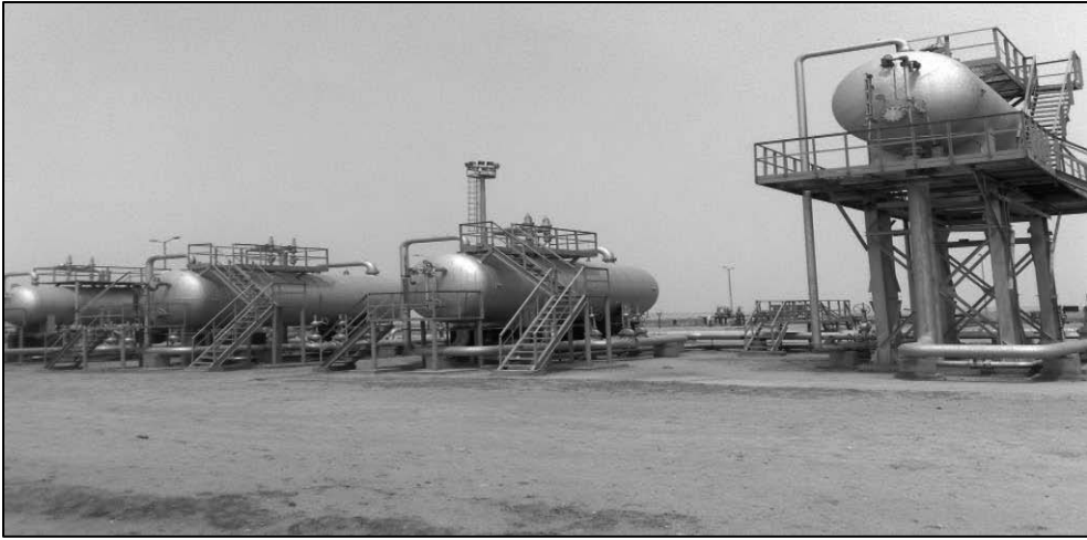
Figure 5: Petroleum Separators, Nasiriyah Degassing Station
