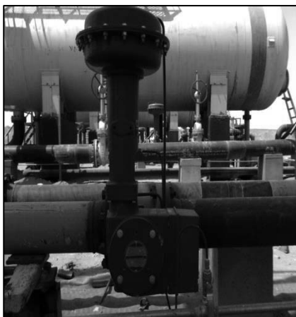
Figure 12: Level Control Valve, Nasiriyah Degassing Station
