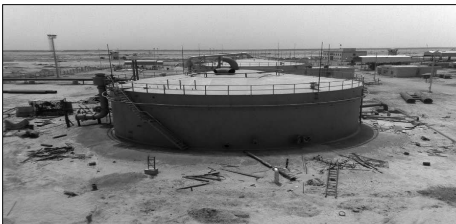
Figure 19: Tank Oil, Nasiriyah Degassing Station
