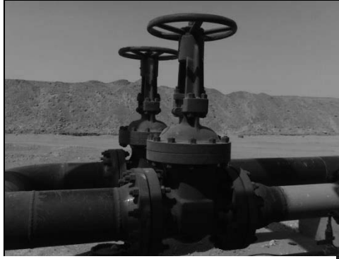
Figure 25: Irreversible Gate Valves, Nasiriyah Degassing Station
