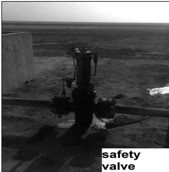
Figure 3: Safety Valve, Nasiriyah Degassing Station
