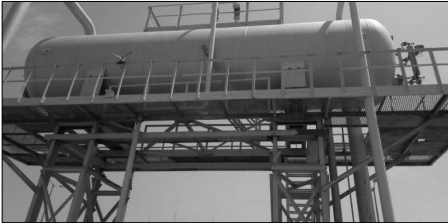
Figure 9: Separator, Nasiriyah Degassing Station
