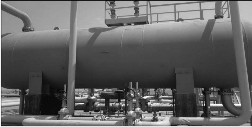
Figure 8: Separator – 1.8 kg/cm 2 , Nasiriyah Degassing Station
