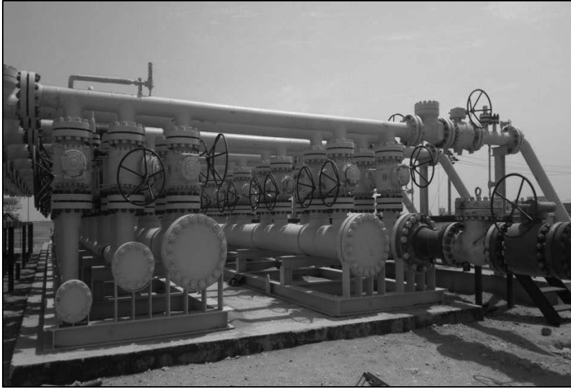
Figure 4: Manifold, Nasiriyah Degassing Station
