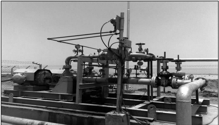
Figure 21: Main Pump, Nasiriyah Degassing Station
