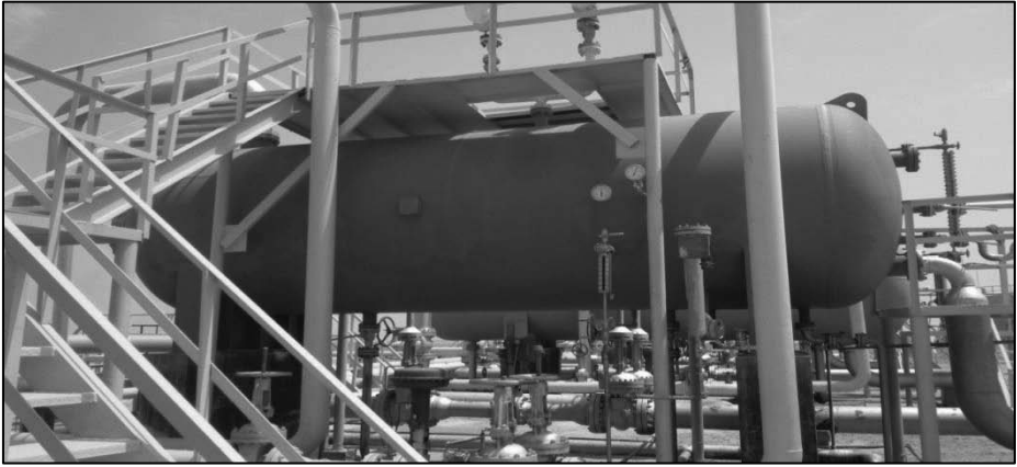
Figure 6: Separator – 28 kg/cm 2 , Nasiriyah Degassing Station
