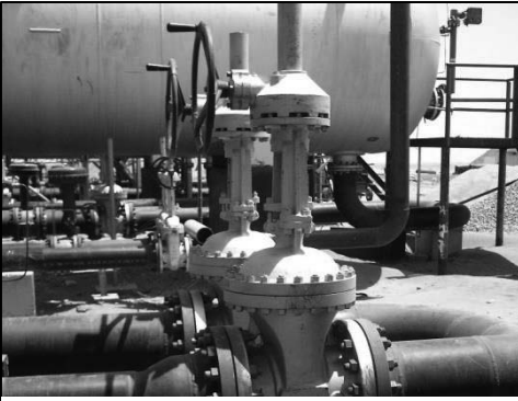
Figure 24: Irreversible Gate Valves, Nasiriyah Degassing Station
