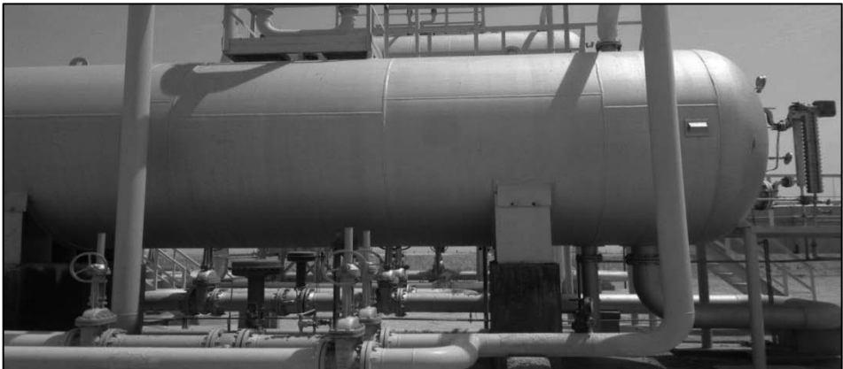
Figure 7: Separator – 7 kg/cm 2 , Nasiriyah Degassing Station
