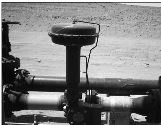
Figure 13: Pressure Control Valve, Nasiriyah Degassing Station
