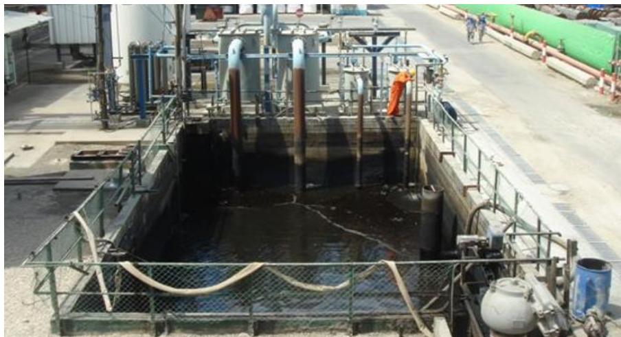
Figure 2: A photograph of a typical API separator at an industrial site.
