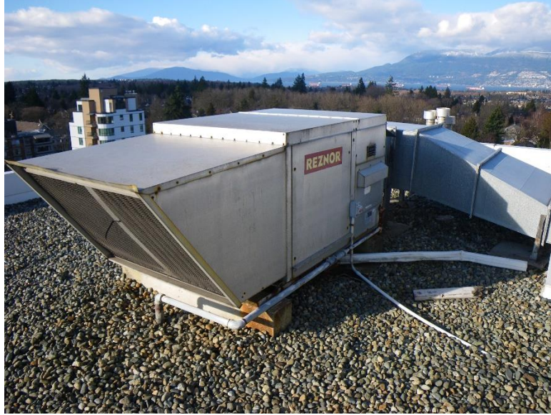
Figure 3-7: The Belmont – Engineered Air rooftop make-up air unit (MAU). Photo courtesy of RDH
