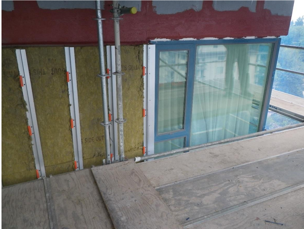
Figure 3-5: Typical exterior wall and new windows during construction in 2012. Photo courtesy of RDH.
