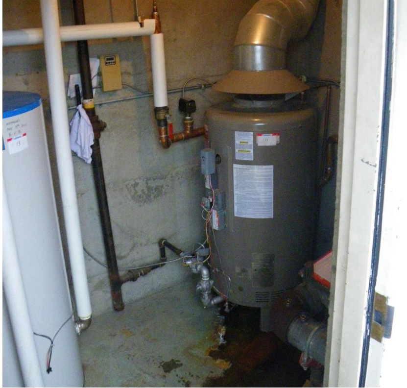
Figure 3-8: The Belmont – A.O. Smith boiler on the left, Allied Engineering Company DHW heater on the right. Photo courtesy of RDH.
