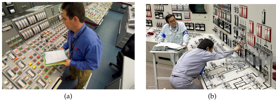
Figure 8.5.: Figure 8.5a shows NPP operator using PBP to train in simulator environments to manage unforeseen emergency events. Figure 8.5b shows operators at Sendai NPP checking the enhanced PBP , introduced by Nuclear Regulation Authority, at a simulator setting in Satsumasendai, Kagoshima, Japan. Source:88.
