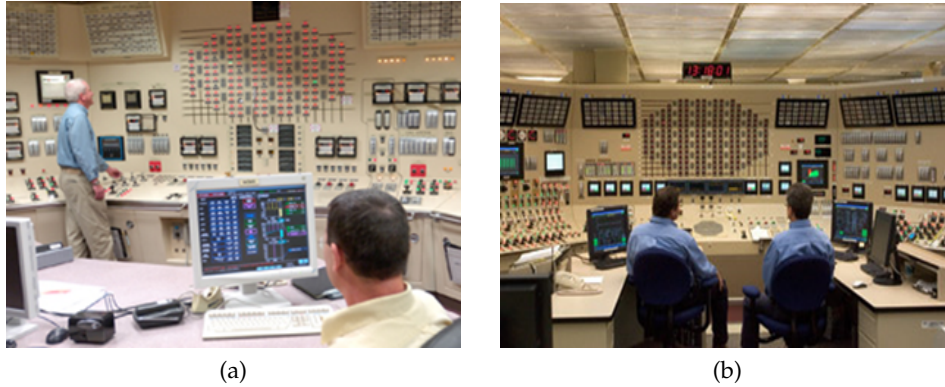
Figure 8.6.: Figure 8.6a depicts a SS interacting with CBP and a RO interacting with the control panel elements. Figure 8.6b shows operators using CBP in a control room at Browns Ferry Nuclear Plant in Athens, Ala., on June 21, 2007. Source:88.
