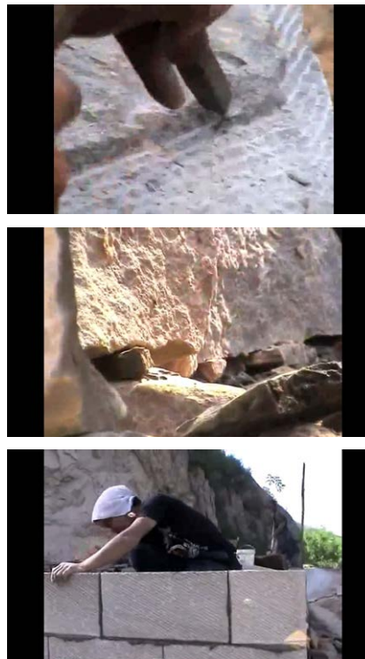
FIG 3.64 Stone-cutting for the facade, Putting the first stones in place, building the walls supporting the vault
