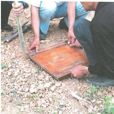
FIG 3.30 Using right angled template to set up the four corners of courtyard
