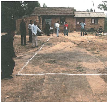
FIG 3.31 Spread white power lines
