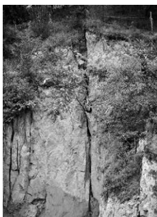
FIG 0.8 A villager checking the cracks of the land after mining have cause land instability in Shanxi Ling-xian Pang-pang-ta village, 2011 Aug.19, photographed by Xin-hua News reporter Zhan-yan
