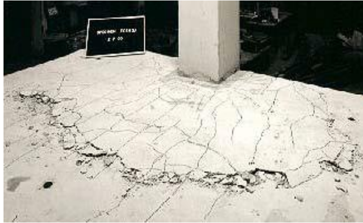
Figure 2.2.4 Cracks after punching shear failure of flat slabs (MacGregor and Bartlett, 2000).
