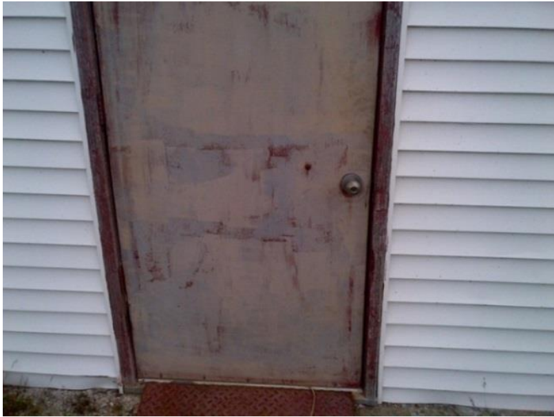
Figure 22: Broken lock to treatment plant
