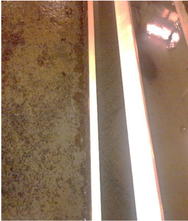
Figure 21: Untreated Water at Treatment Facility
