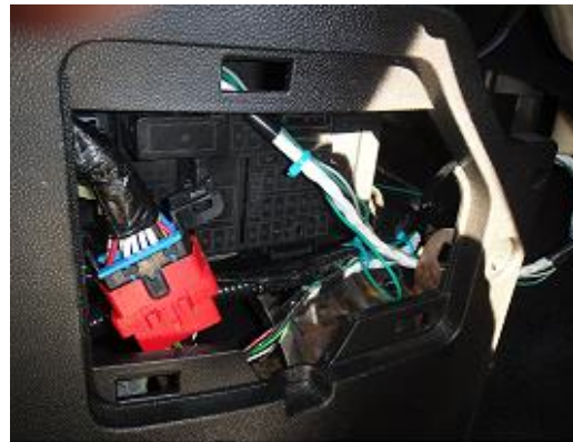
Figure 4-4: Data logger connection and shut down wire
