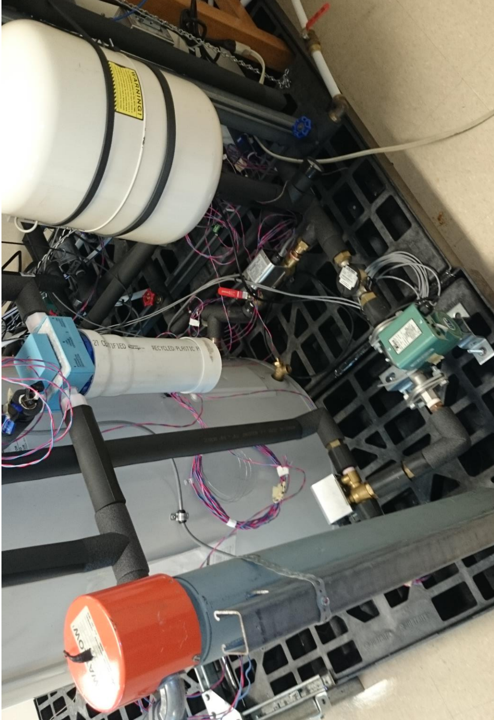
Figure A.3 – Electrical resistance heater (left), expansion tank (right), source-side hydronic pump (bottom), water filter (top)
