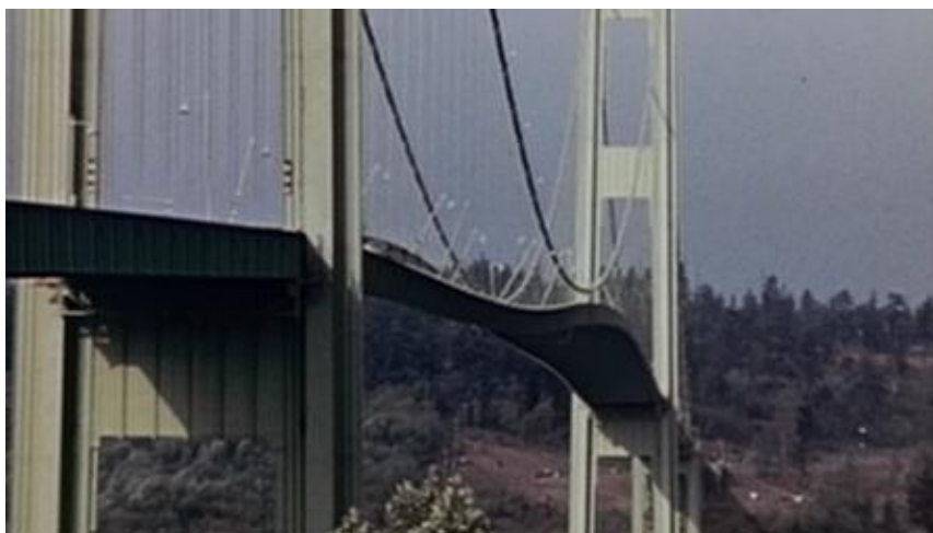
Figure 2.1 Destruction of the Tocomas Narrow Bridge ( http://en.wikipedia.org/wiki/Tacoma_Narrows_Bridge-1940 )
