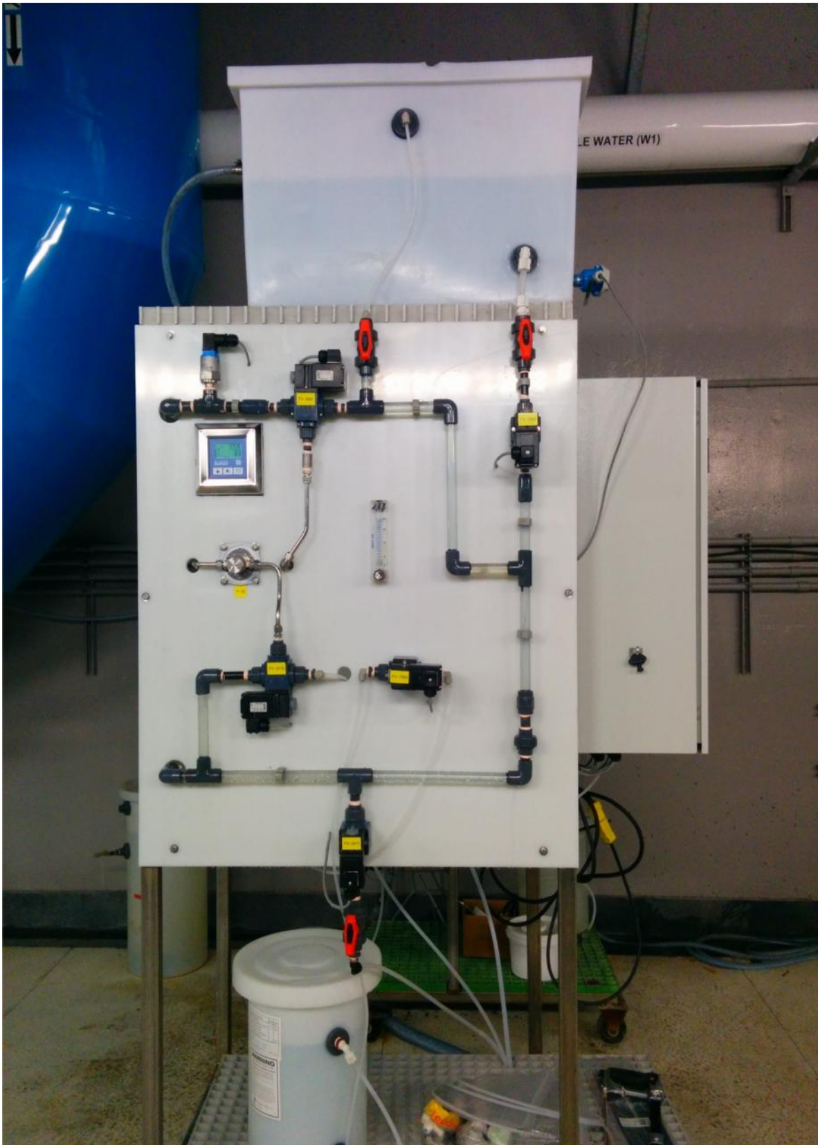
Figure A-3. UF Pilot#3 side view showing mechanical and electrical components
