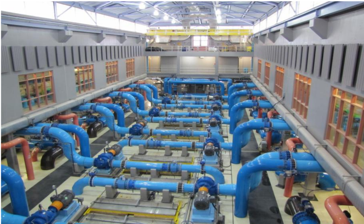
Figure 3.3 Membrane effluent treatment pipes at the Lakeview WTP
