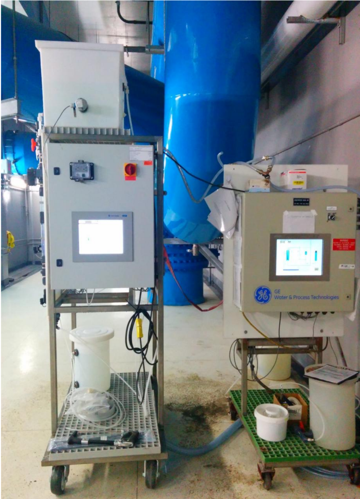
Figure A-5. UF pilot#1 (right) and #3 (left) in parallel operation
