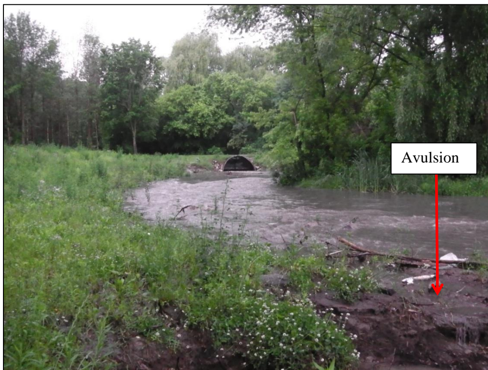
Figure 67. Failing restoration in upper reach of Section 2.
