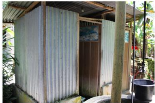
b) Shared bathroom facility in Kategan
