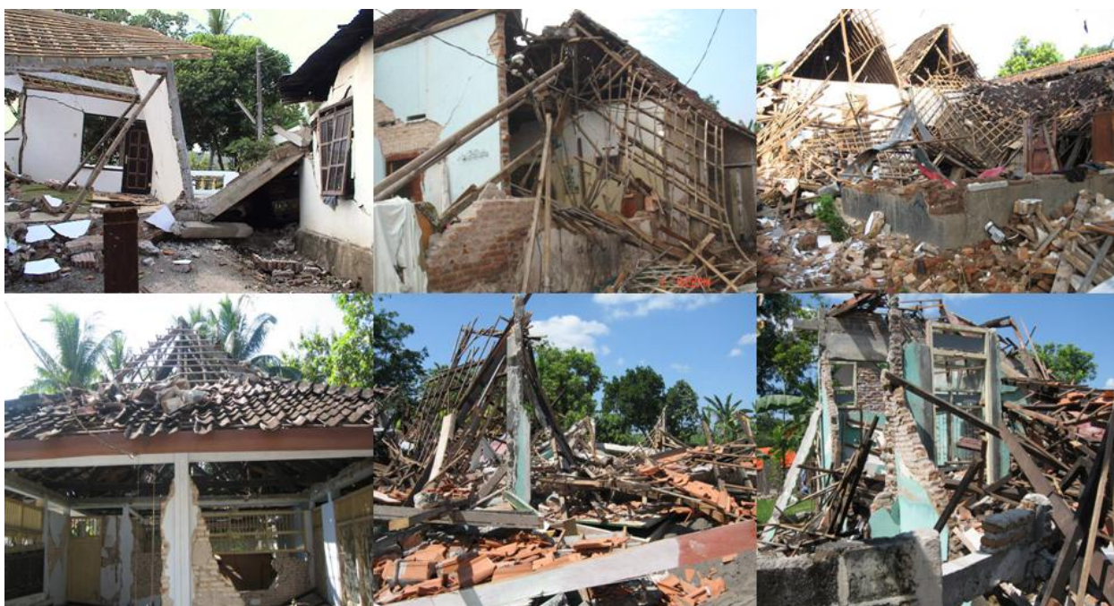
Figure 4.4: Structural Failure of Walls and Roofing in Private Dwellings
