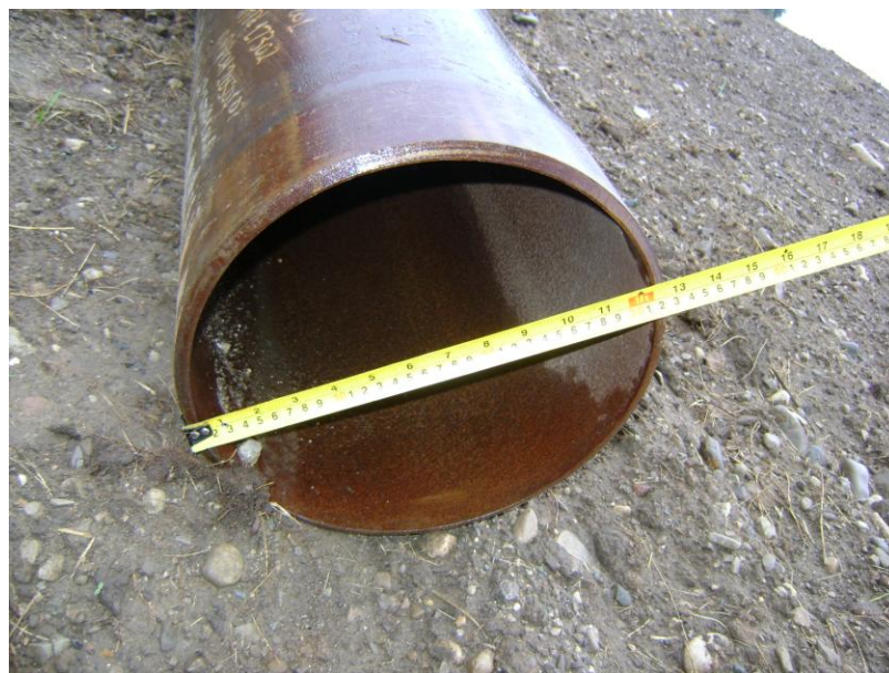
Figure 3-8: Steel Conduit Used for Cable Crossing
