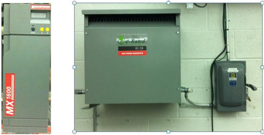
Figure 3-31: MX 1600 driver and 460V 3 phase transformer.
