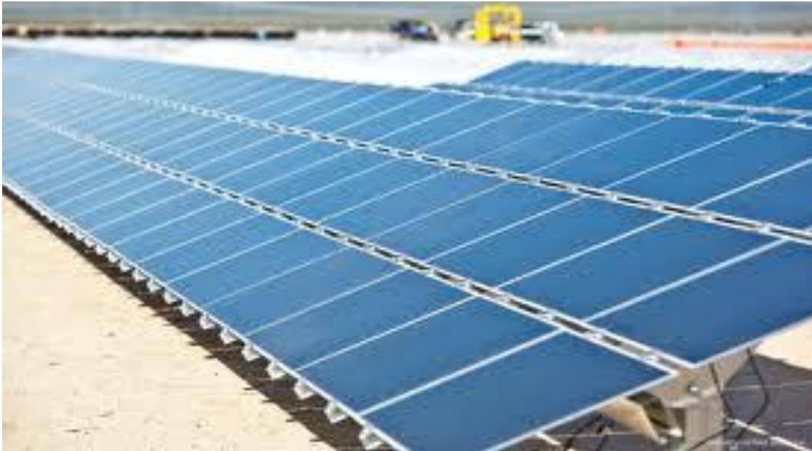
Figure 1-7: A PV farm installed in portrait to reduce installation cost
