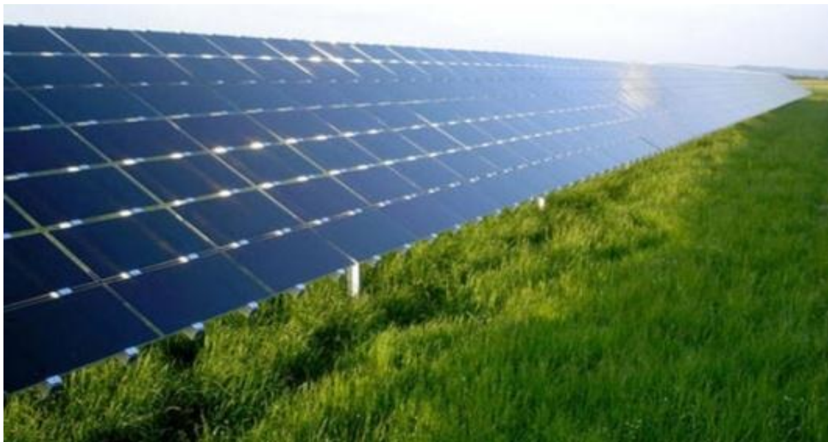
Figure 1-8: A PV array which large number of rows to reduce installation cost
