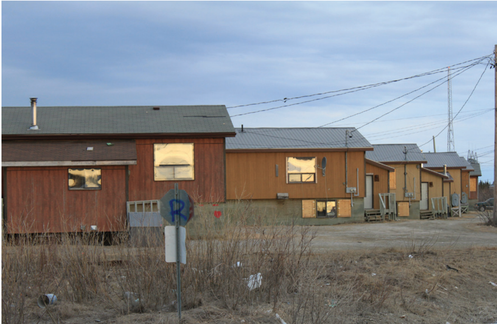
Fig. 31 - One row of the teacher's housing. The reflectivity of the windows is caused by the sheets of plexi-glass that are screwed overtop the exterior frame in an effort to protect the windows from rocks and other objects thrown by kids. This is a huge fire safety issue.
