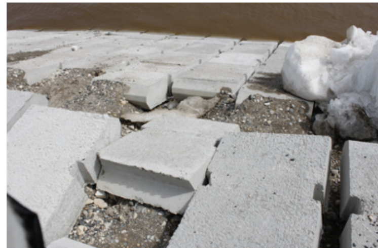
Fig. 29 - Many of the blocks along the lower edge have been dislodged by the massive ice chunks. None of the blocks are tied back to the dike, they just rest on the surface.
