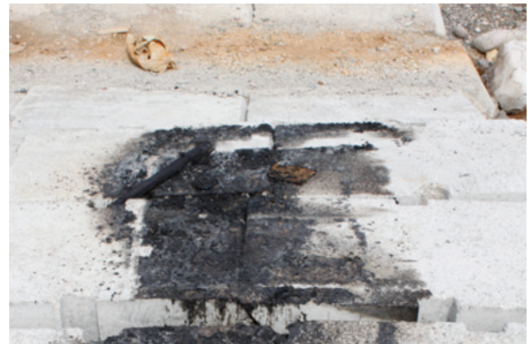
Fig. 72 - Charred remains left by an unknown source on the concrete blocks lining the edge of the dike.
