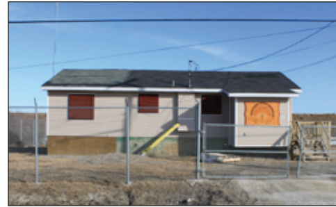
Fig. a238 - Kashechewan Power Corporation building
