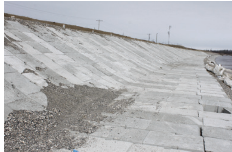
Fig. 28 - Concrete blocks, installed in 2010, protect the dike from yearly erosion. This image shows the dike after its first winter. Many blocks have shifted but the overall system seems to be functioning as intended.
