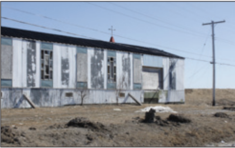
Fig. a2 - Abandoned old church
