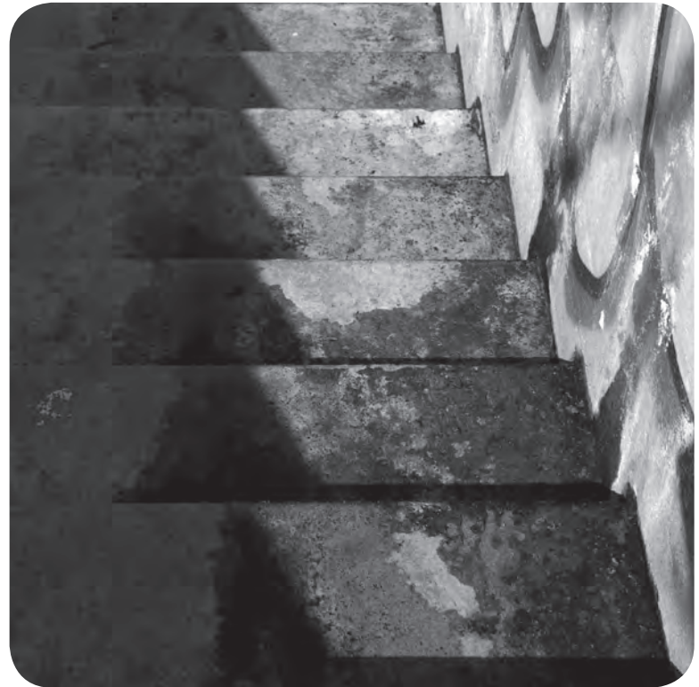
fig. 1.89 'Puddles' on the stairs down to the river.
