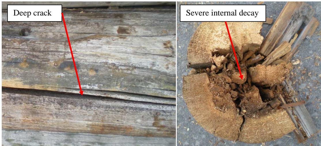
Figure 72. - In-service specimen with deep crack and severe decay (D-1-1).
