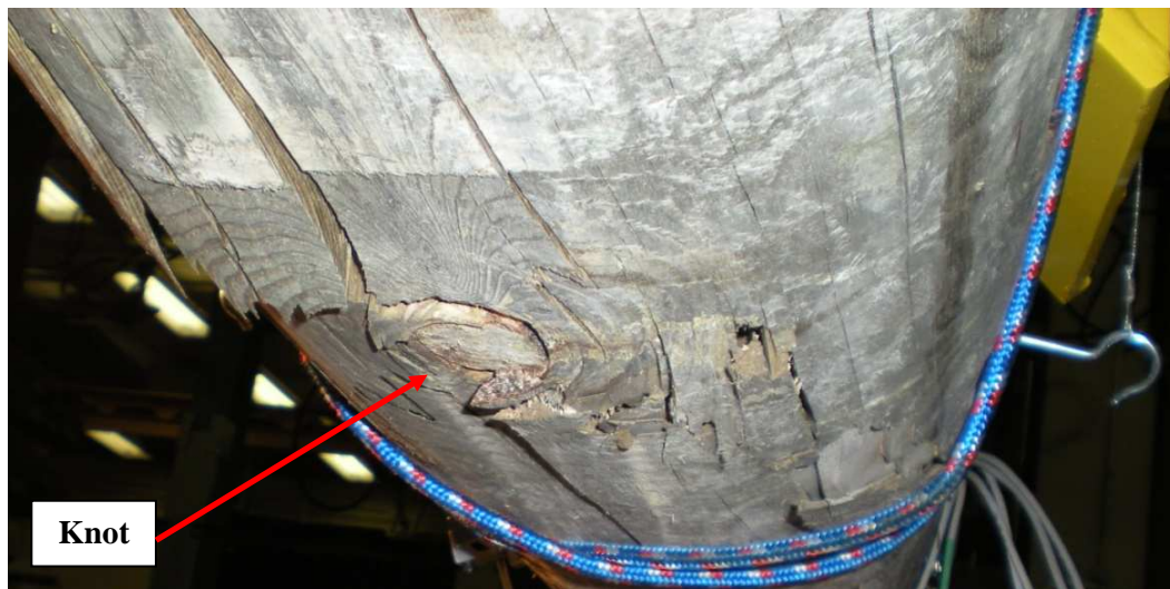
Figure 37. - New pole specimen with a large knot at failure location (45-1-2).
