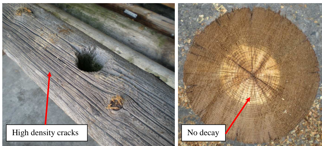
Figure 73. - In-service specimen with shallow and high density cracks with no decay (D-2-1).
