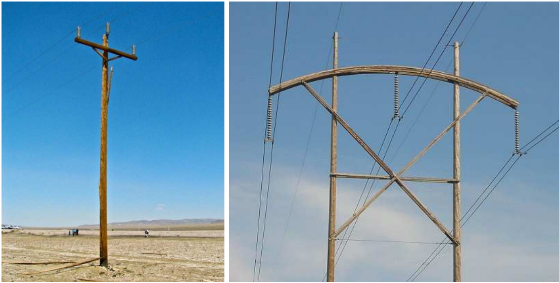
Figure 1. - Electrical distribution and transmission structures constructed of wood utility poles.
