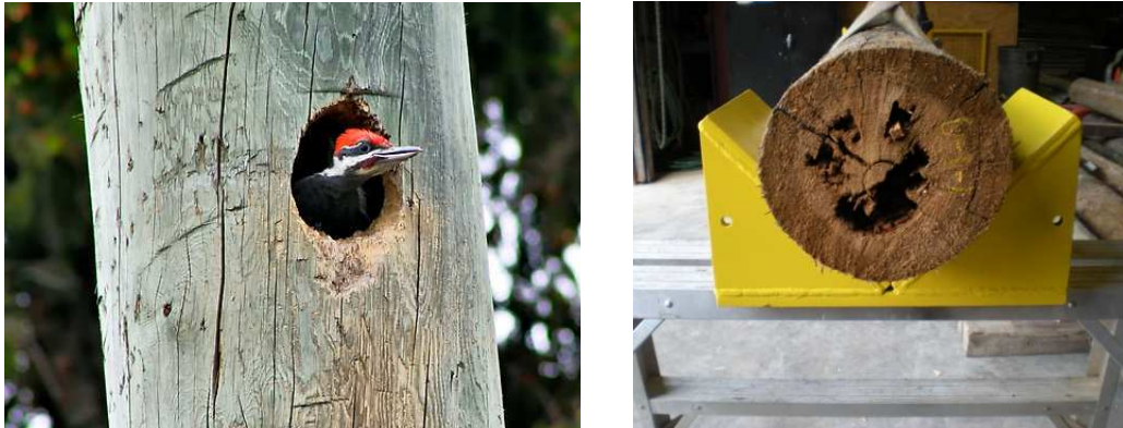
Figure 2. - Woodpecker damage (left) and decay (right).
