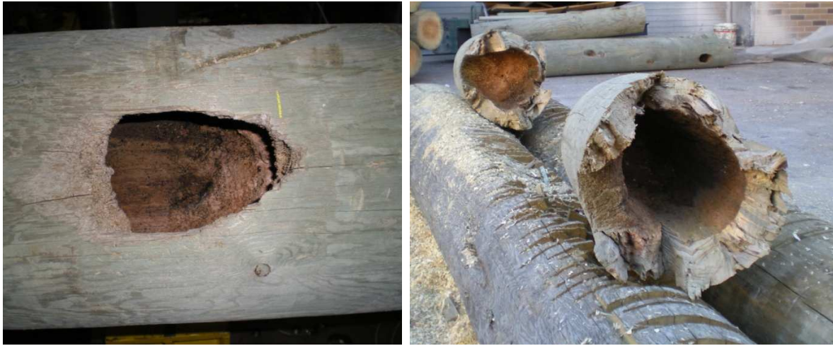
Figure 11. - In-service nesting damage and dissection of interior.
