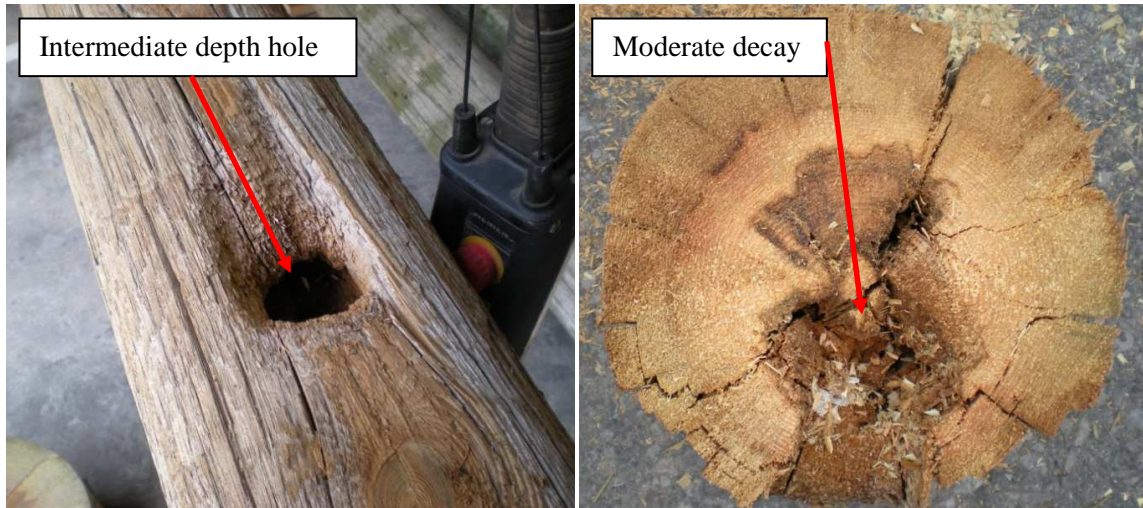
Figure 76. - In-service specimen with intermediate level woodpecker damage and decay (D-3-1).
