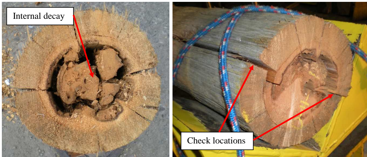
Figure 83. - Heavily decayed in-service specimen that failed in shear (D-4-1).
