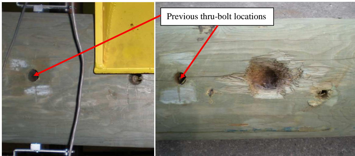
Figure 80. - In-service specimens with mechanical damage and no decay (60-4-2).
