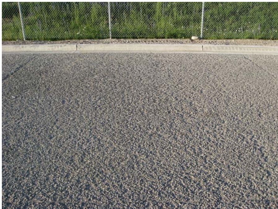
Appendix A-8 Surface Distress Rating: Fair (Overall View).
