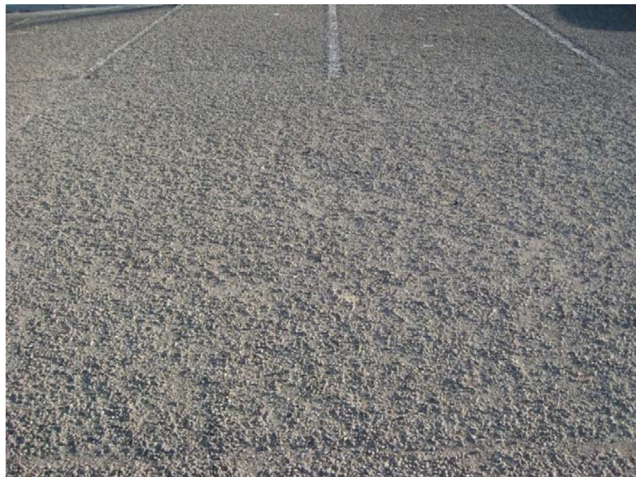
Appendix A-10 Surface Distress Rating: Poor (Overall View).
