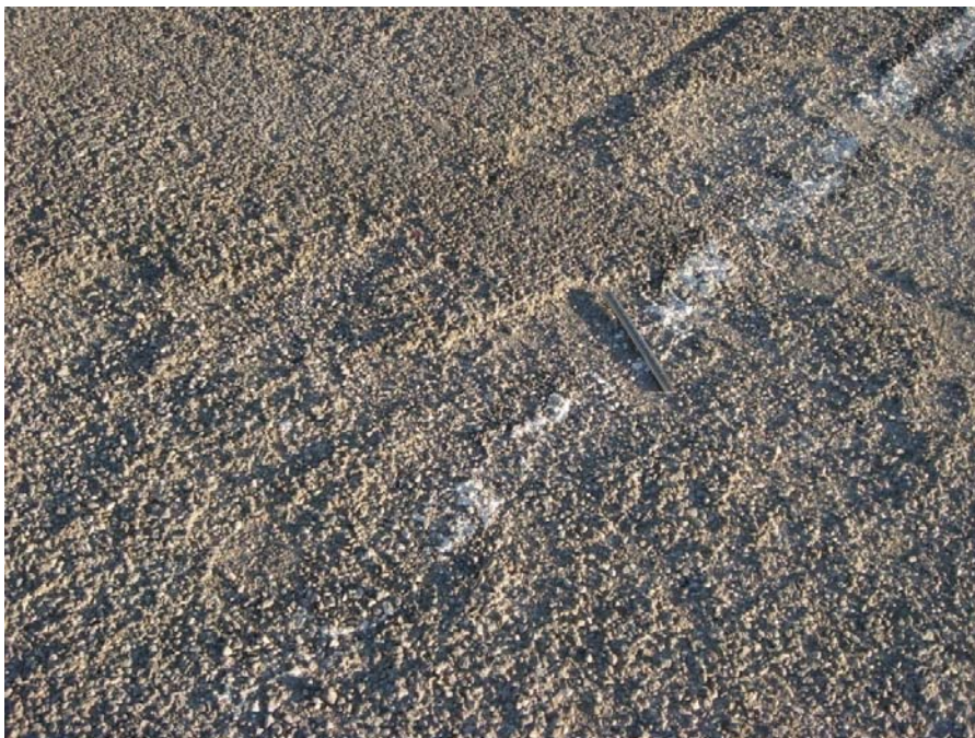
Appendix A-12 Surface Distress Rating: Very Poor (Overall View).
