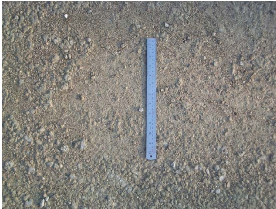
Appendix A-11 Surface Distress Rating: Very Poor (Close View).
