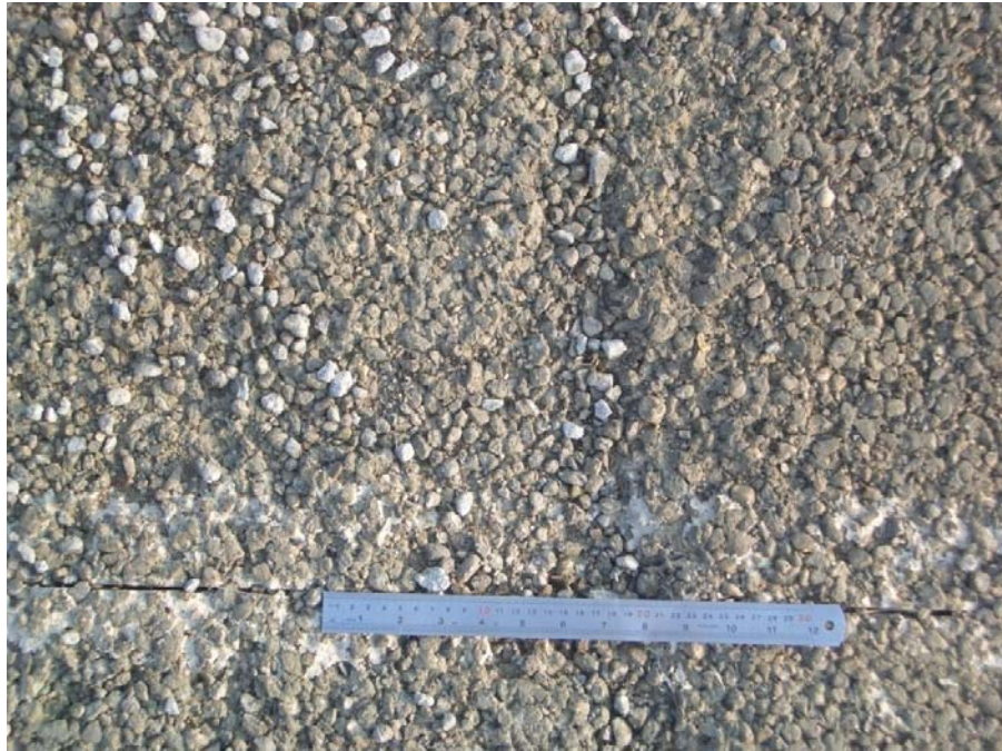
Appendix A-9 Surface Distress Rating: Poor (Close View).
