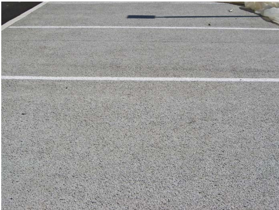
Appendix A-4 Surface Distress Rating: Very Good (Overall View).
