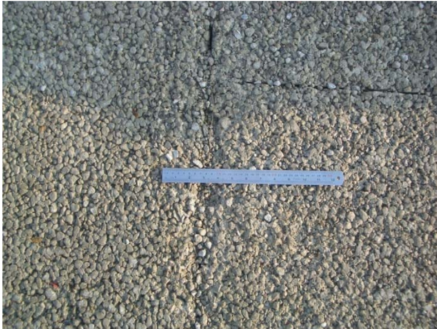
Appendix A-7 Surface Distress Rating: Fair (Close View).
