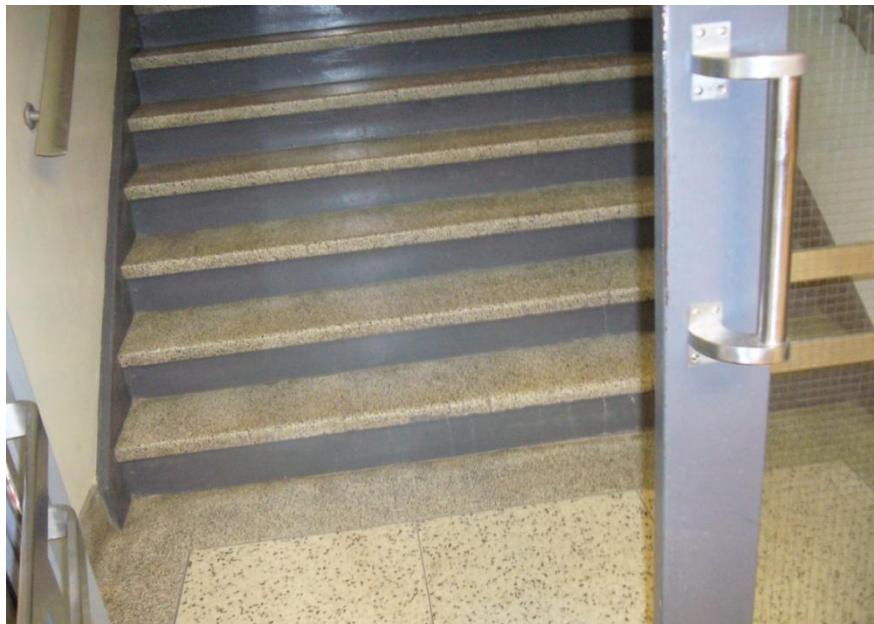
Image 3: Inaccessible Access to the Fitness Centre Lacks Signage of Accessible Route
