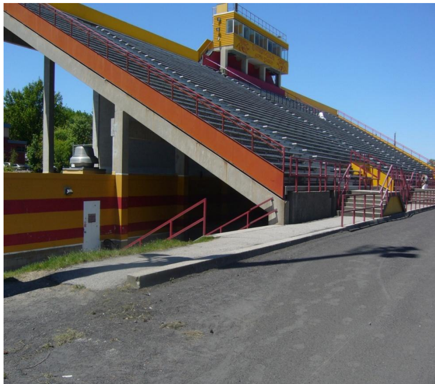
Image 6: Ground Level Accessible Spectator Area Blocks Stairwell
