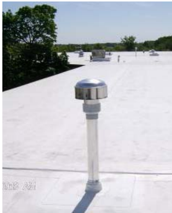
Figure 6-5: Passive vent pipe
