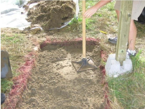
Aug. 21 st , 2008 (day 0) – WT = 52cm bgs: Trench packing after E10 spill. Red stain on the sides indicates that some of the gasoline infiltrated through the sides of the trench.
