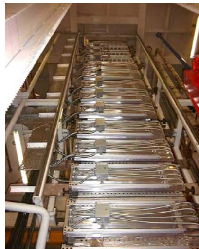
Figure 5.14 View of the Clydach Foam plant plating column
