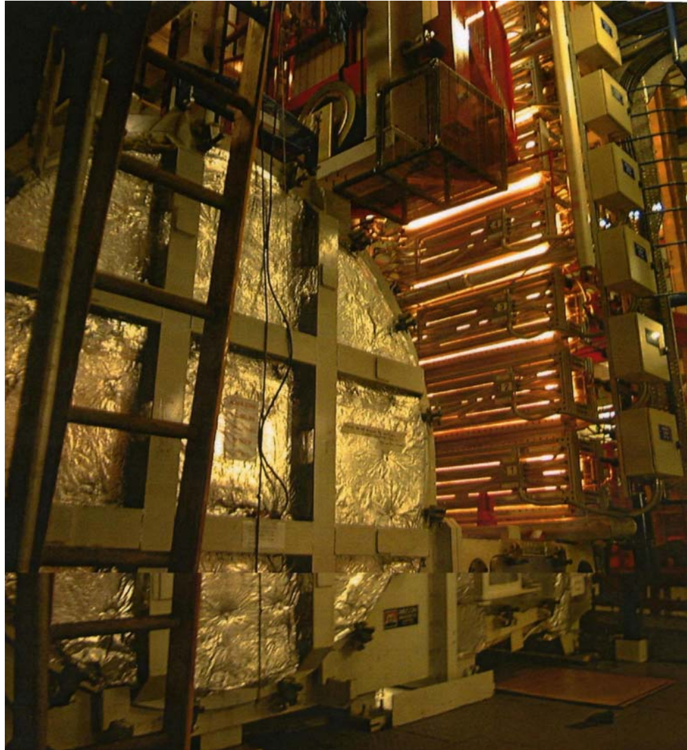
Figure 5.16 Uncoiler and the lower chambers of the commercial foam plater in operation (Vale Inco Europe Nickel Refinery 1999-2006)
