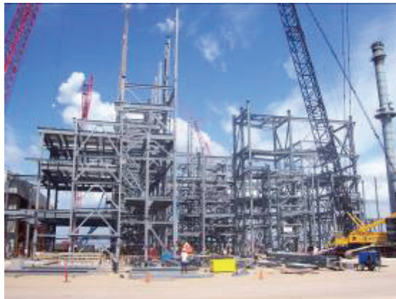
Figure 4.18: Boiler structure, Rockdale, Texas, USA
