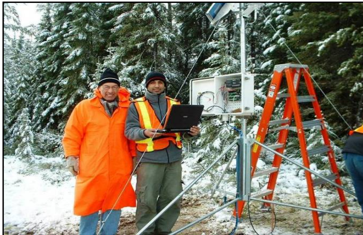
Figure 4.9: Sensors installed, Tower Erected, Data logger Programmed and the set up is being tested on Hwy 651
