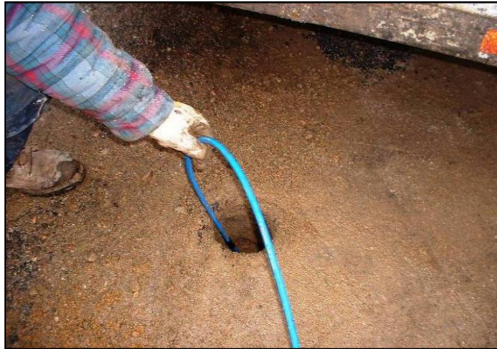
Figure 4.3: Thermistor String Installation Backfilled with the same material, rammed, and sealed with cold mix. (Hwy 651, Nov. 6, 2007)
