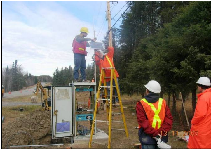
Figure 4.10: Erection of Campbell's Tower arrangement eliminated and the mast is being fixed to the Cabinet provided by MTO, Hwy 601
