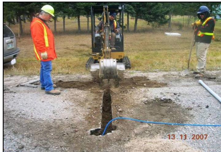
Figure 4.4: The saw cut trench is ready for the string to go in, Hwy 601
