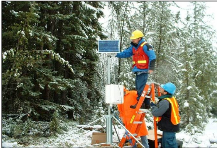
Figure 4.8: Tower mounted with Data logger Cabinet and Solar Panel, Hwy 651
