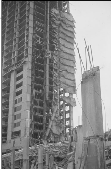
Figure 1.4 Collapse of Skyline Plaza (adapted from Building Science Series 179, 2003, by Building and Fire Research Laboratory of the National Institute of Standards and Technology, USA)
