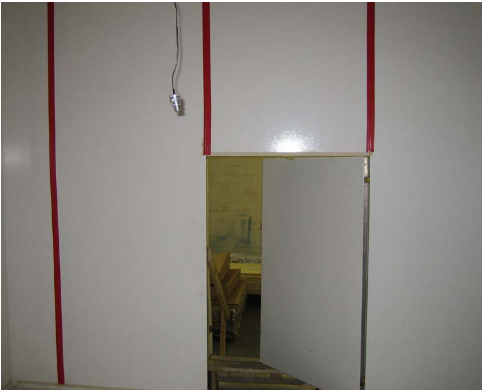
Figure 3.5: Chamber Interior, Back, Left and Front Wall with Door
