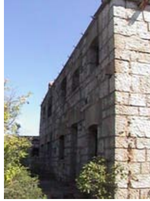
Fort Klinci Fig. 4.26 (left) The access road and the surrounding context Fig. 4.27 (right) The entrance and the north facade
