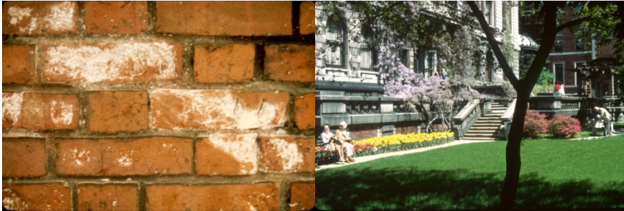
Figure 2: Detail of the brick wall showing the gypsum efflorescence formed on the parallel wall below grade to that seen in the garden at right.
