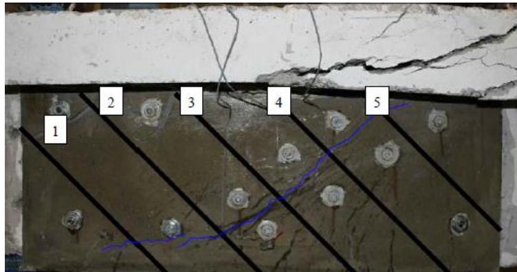
e) Crack pattern in the lateral surface of T-D-5L-BC beam at failure load
