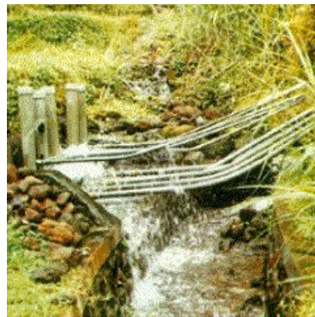
Figure 6. Installation of More than One Hydram Pump in Parallel Way
