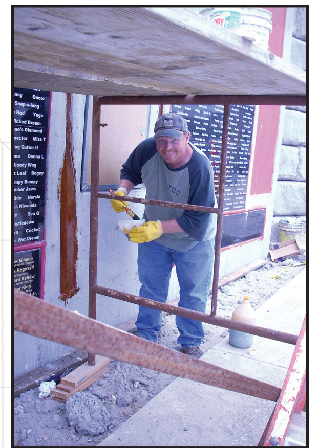
Mason and doryman Richard Bush stains the oars, which are molded into the concrete, before applying a beige slurry to "finish" the wall.
