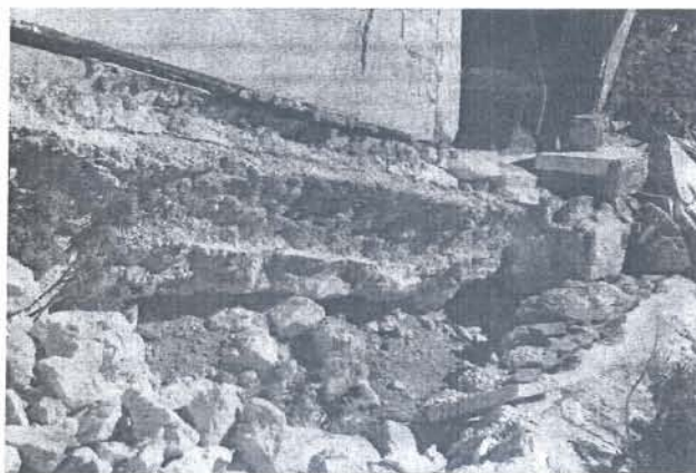
Fig. 12. Shallow foundations in deluvium mass which moved as a cause of overturning
