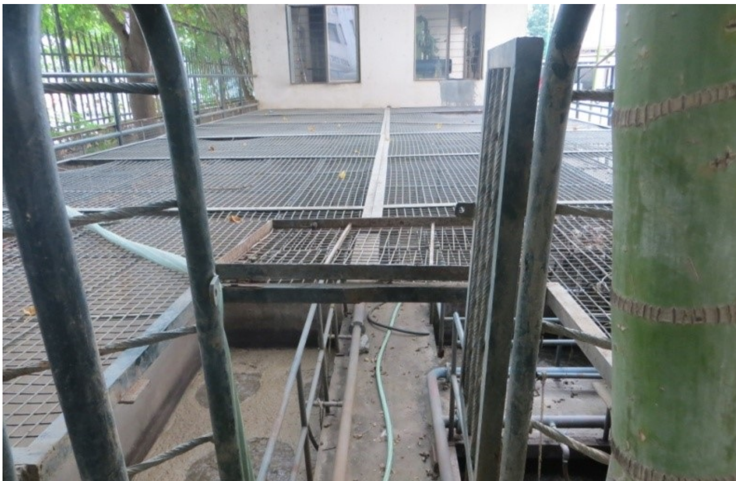
Aeration tank of an STP employing the Activated Sludge Process (ASP). Pic courtesy: ATREE
