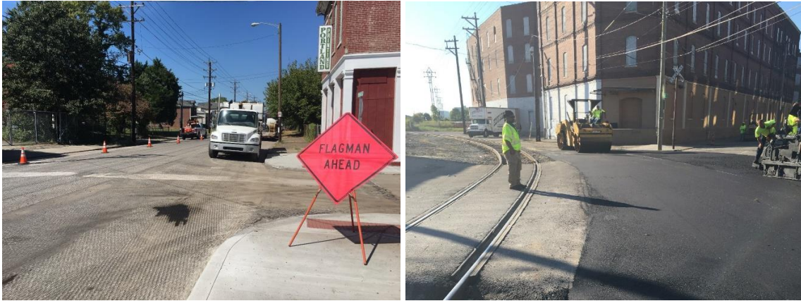
Fig. 5.8. Field view of mill and overlay on Portland Avenue in Louisville, KY
