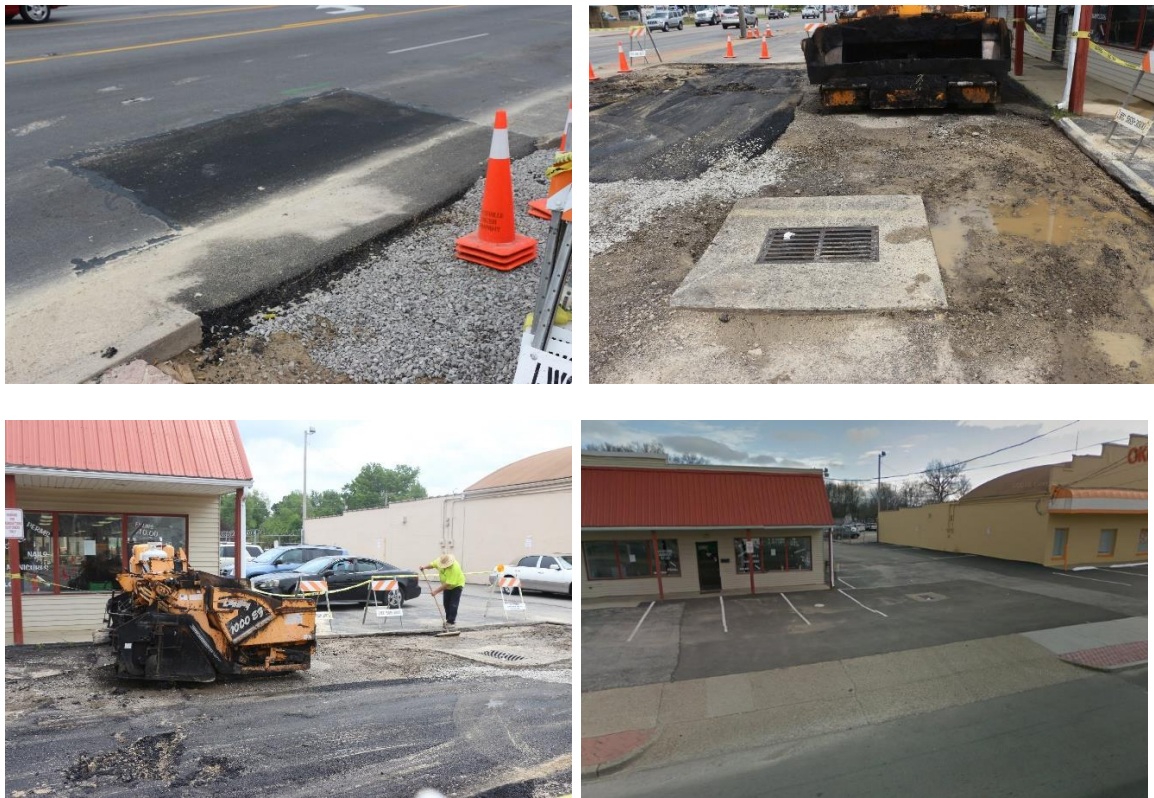
Fig. 5.3. Field view of utility cut restoration on Preston Highway in Louisville, KY
