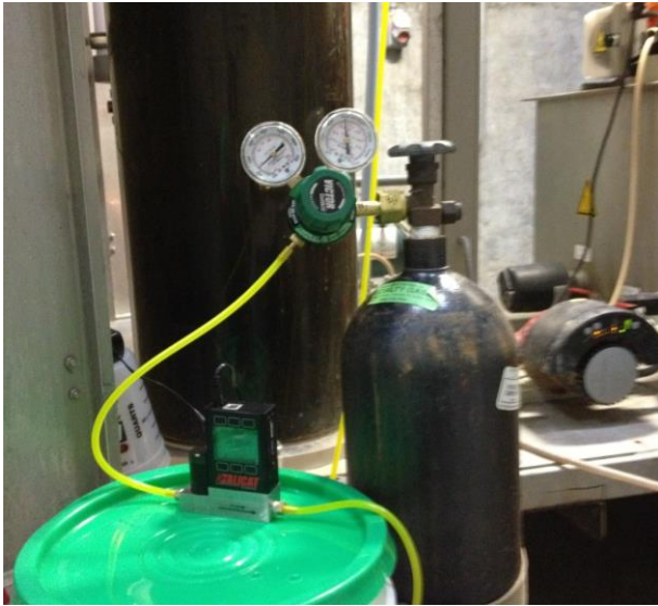
Figure 3-5 Gas flow controller setup to inject the hydrogen gas to the main reactor
