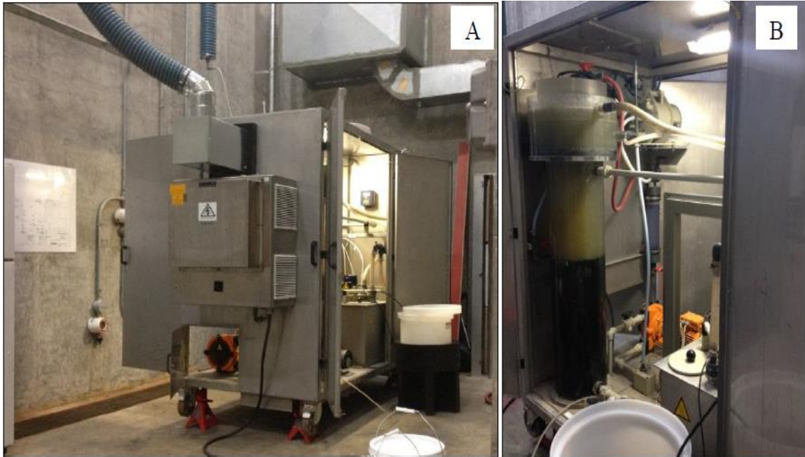
Figure 3-2 (A) 60 liter continuous up-flow AD reactor system; (B) Main AD reactor
