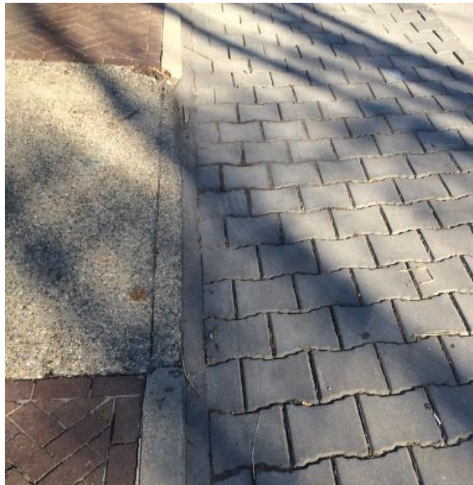
Figure 20. PICP 19H (a) Upgradient edge (b) Curb Condition
