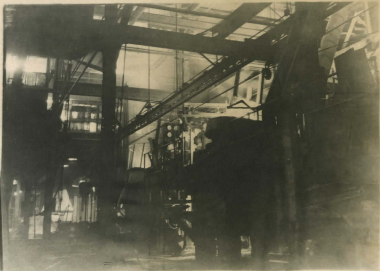
Fig. 5. Electro-cast furnaces - one hooded (in foreground) one unhooded (in background)
