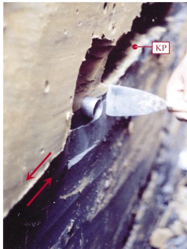
Fig. 6 Sampling in the immediate vicinity of the slip plane (KP) in drain "6" (Photo by V. Belošević, May 7, 1998).
