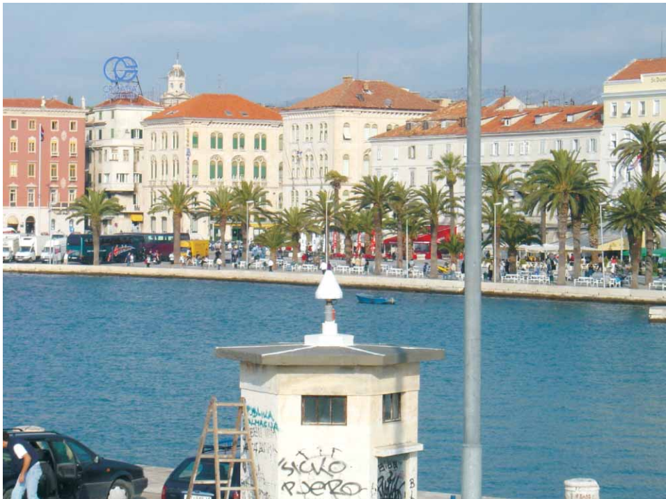
Figure 15. The photo of CGPS antenna mounted on top of the roof of the Split tide gauge.
