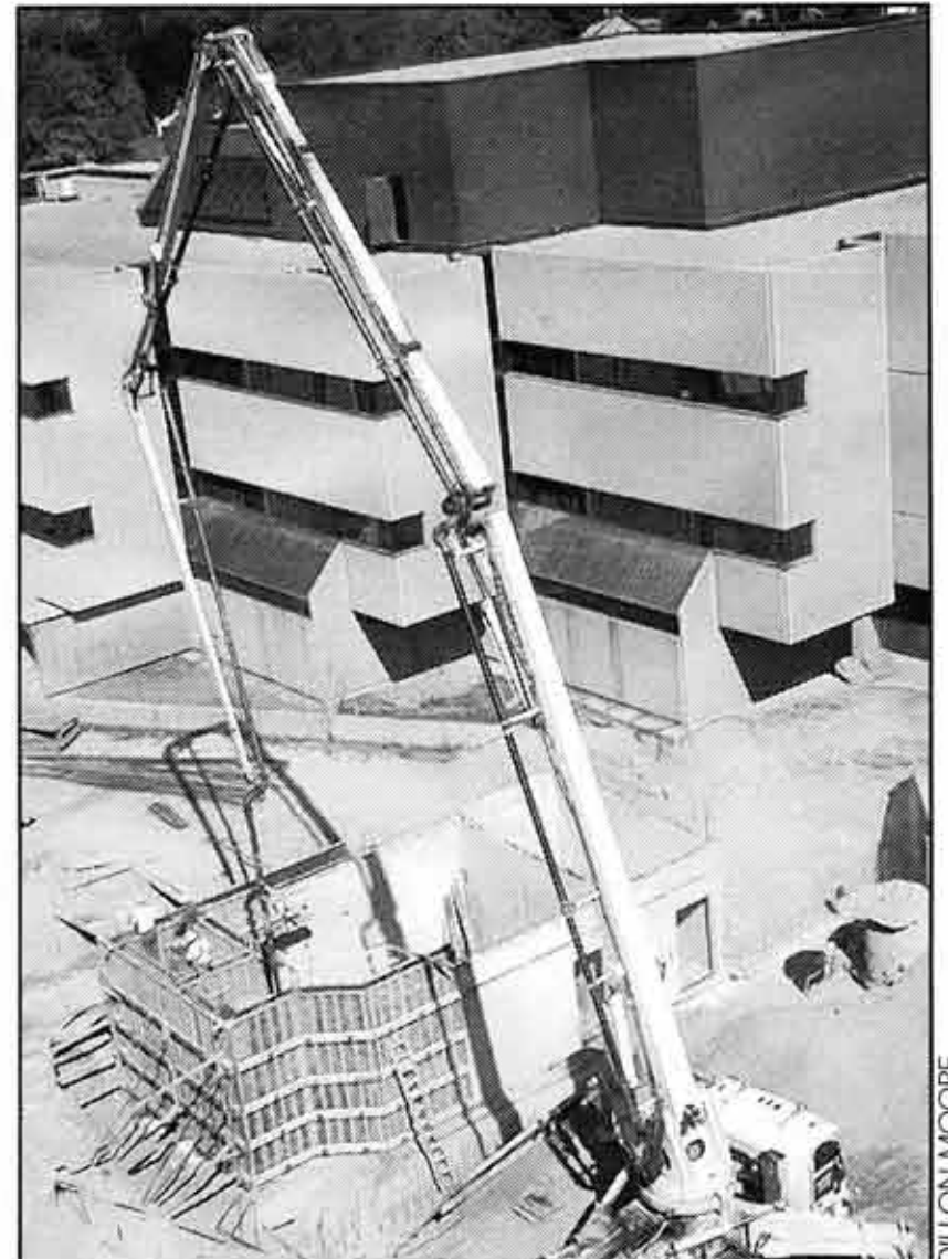
Wilfrid Laurier's campus is in shreds with construction, as the university prepares for a dramatic increase in students.
