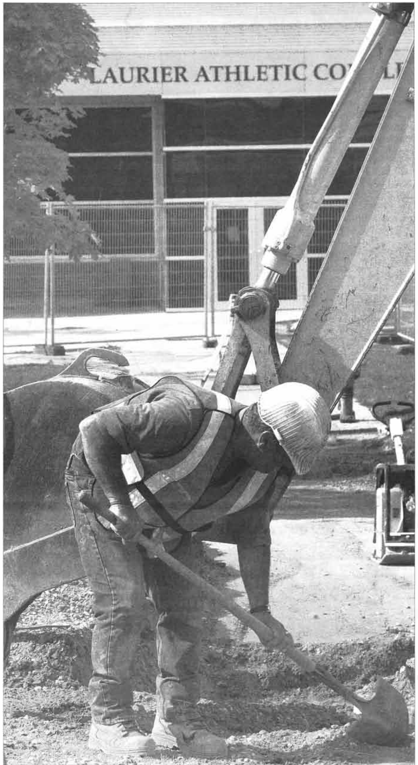
MAN AT WORK - Work along the exterior of the AC to improve water drainage will be completed this week.
