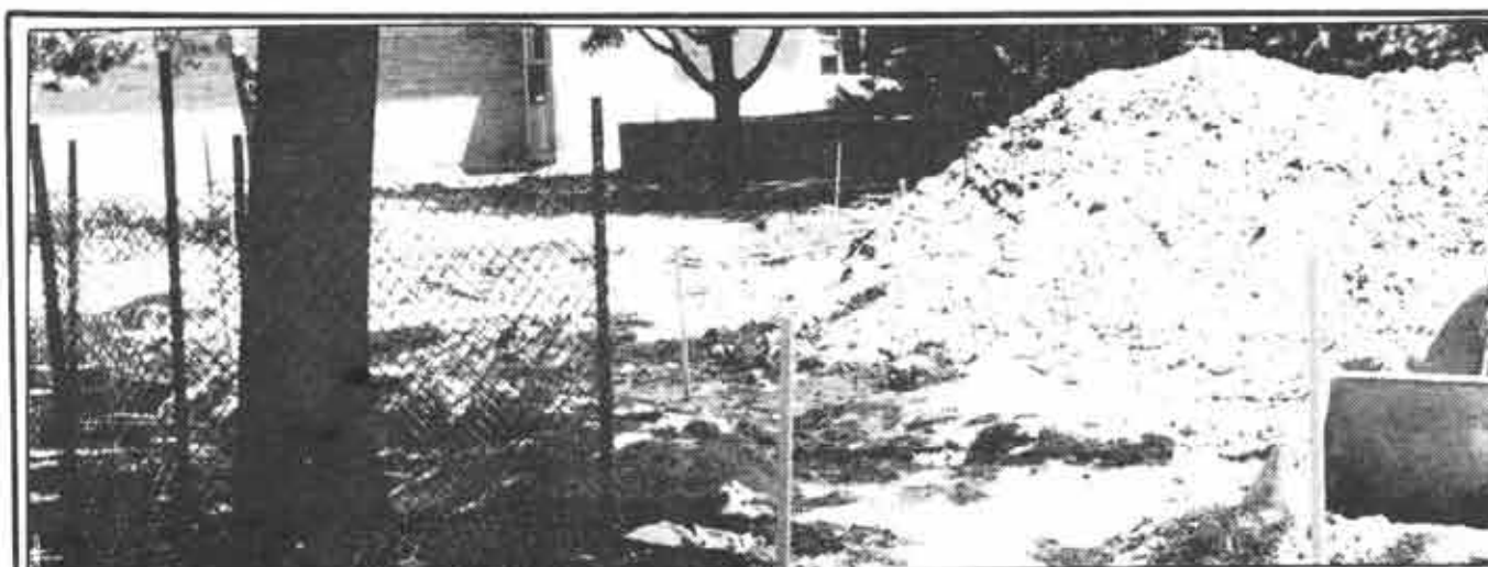
Summer's here and so are the bulldozers. It's construction time at Laurier where they try to make our campus look better. First they have to clear away all the buildings and transpose some of Westerns buildings over here. (Ooooh, blasphemy!)
