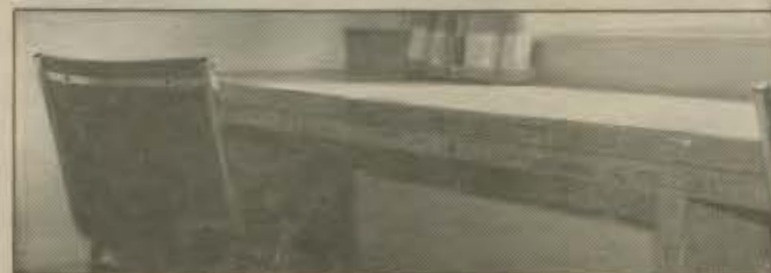
More B3 damage. Cute writing on the desk and chair is typical of every room. The whole place needs to be repainted as well.
